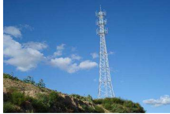
Remote communication base station, fiber to the tower (FTTA).
