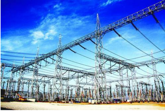
Intelligent substation control system
